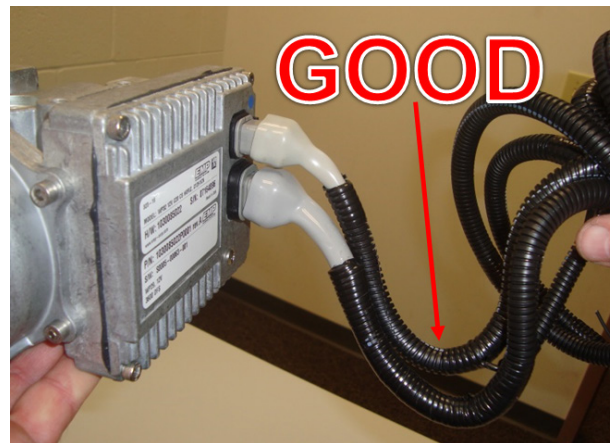
Good Wiring – Drip loops
