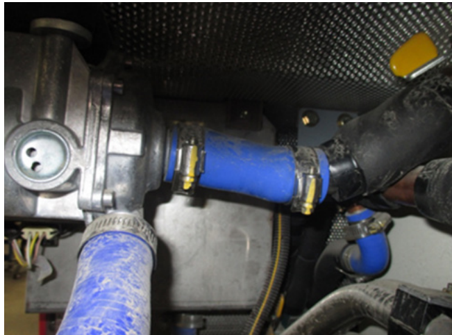
Improper installation with localized high spots
